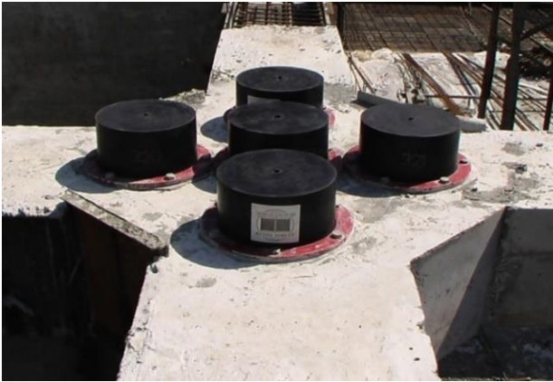
Fig. 1. Layered rubber bearing seismic isolators used in Armenia [4]
